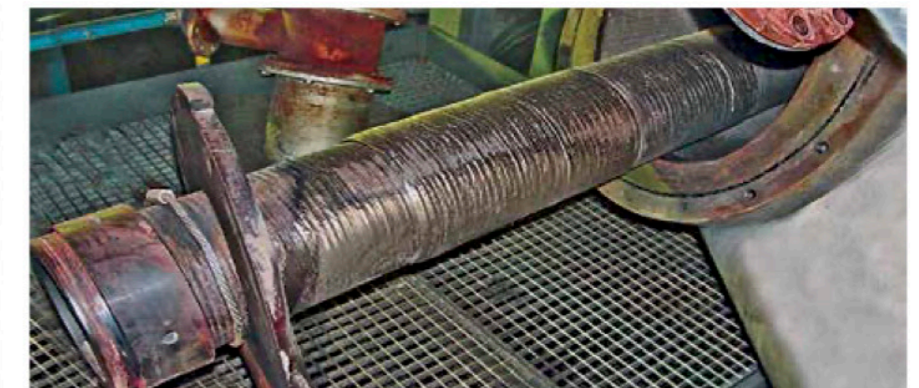
PF-burner lined with KALMETALL.
