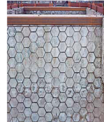
Extended service life of plant components
