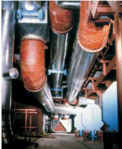
A typical application in power plants is pulverized fuel piping.
