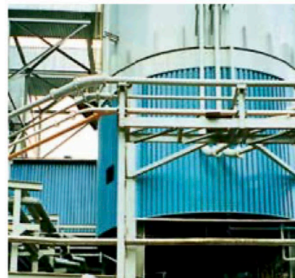
Limestone may have a very abrasive effect in FGD systems; a typical lining material is ABRESIST.
