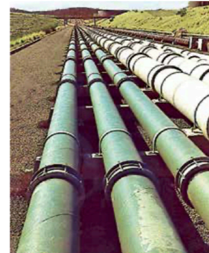
Wear protection for hydraulic and pneumatic pipes
