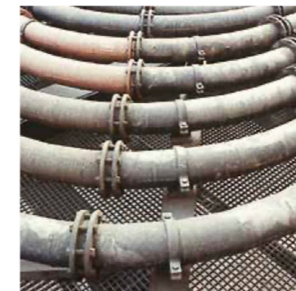
Extended service life of plant components
