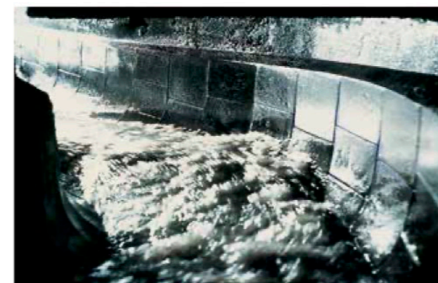
Scale launders are effectively lined with ABRESIST fused cast basalt
