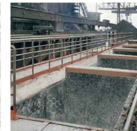
Hydraulic and pneumatic pipes
