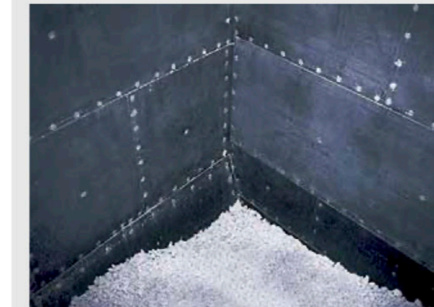
Limestone bunker with slide promoting lining made of KALEN 1006
