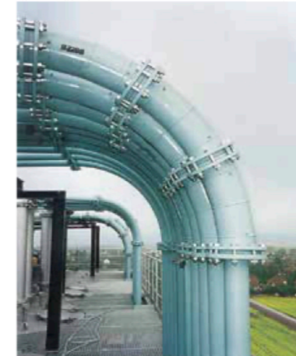
Protection for pneumatic and hydraulic pipes
