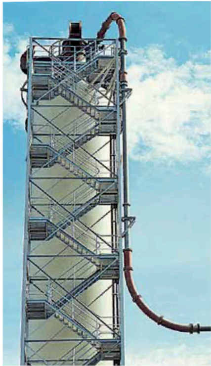
Transport pipe to the cement silos; the bends are protected by ABRESIST
