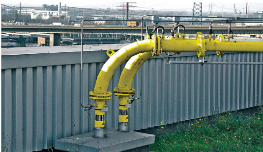
KALDETECT equipping a German waste incineration plant
