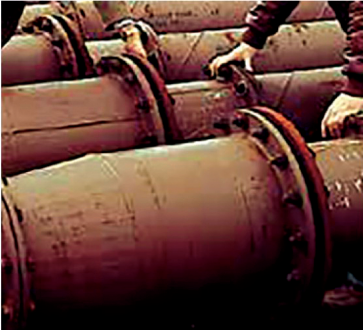
Expansion joint in a hydraulic ash line
