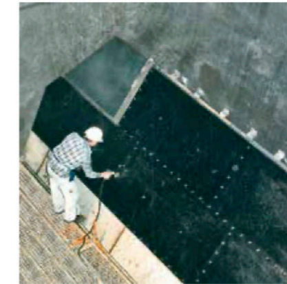
Large bunkers are efficiently and reliably lined with KALEN slide promotion plastics.
