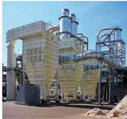
The fine dust that occurs in processing plants is extremely abrasive. This requires the plant components to be carefully protected. It is done both with metallic and ceramic materials.
