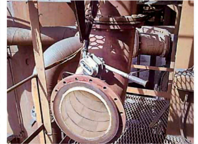
Pipes protected with KALCOR zirconium corundum installed in the discharge section of an iron ore grinding mill in Brazil. Rubber linings failed after a few months whereas the KALCOR lining has been in operation for several years.
