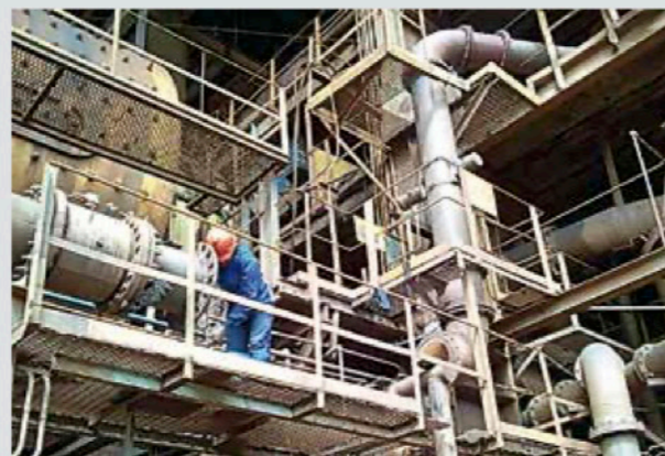
In Brazil the rubber lining in the pipe from the grinding mill to the classifying of the iron ore failed after a short time. These pipes are now lined with KALCOR zirconium corundum.
