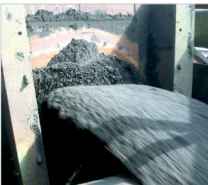
KERFALEX lining of a bin set up in a bulk material handling plant
