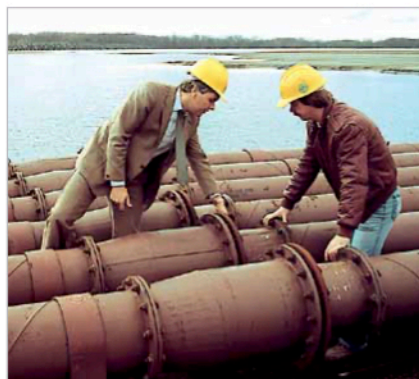
Expansion joints in a hydraulic bottom ash pipeline
