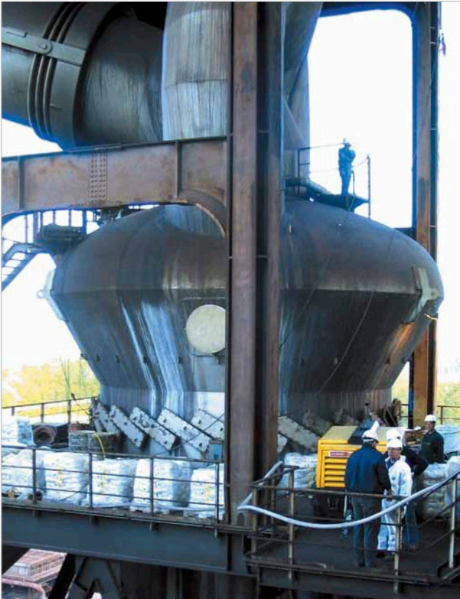
Scrubber inlet in a steel plant lined with sprayed-on KALCRET-BTS hard compound
