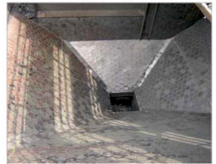
Coke bunker in the iron and steel industry
