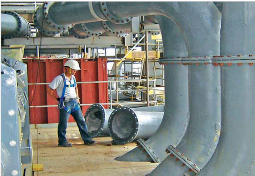
Typical applications of KALMETALL-C hard casting are pipe systems; here a pulverized coal pipe of a power station in South East Asia
