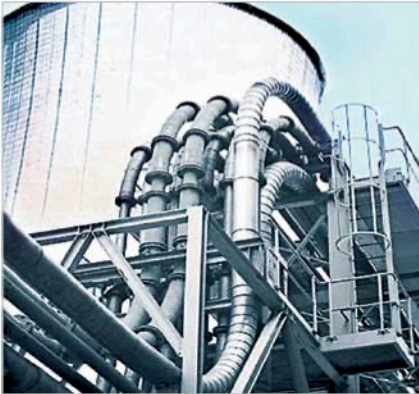
Fly ash pipelines in a coal fired power station
