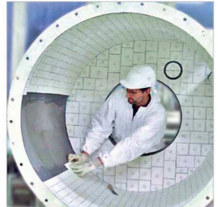
Lining a cyclone inlet with KALOCER; the arch shape enables fixing radial shaped elements in KALFIX setting compound whereas the headwall requires mechanical fixing by means of weld sleeves and ceramic caps
